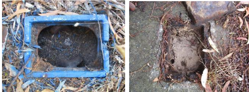
Figure 4: Examples of Silted Up FPs
